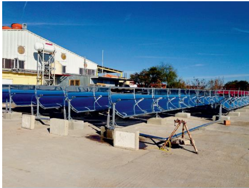
Fig. 2.3. Application of parabolic trough collector in a dairy processing plant in Mexico (Kasibhatla, 2015).
