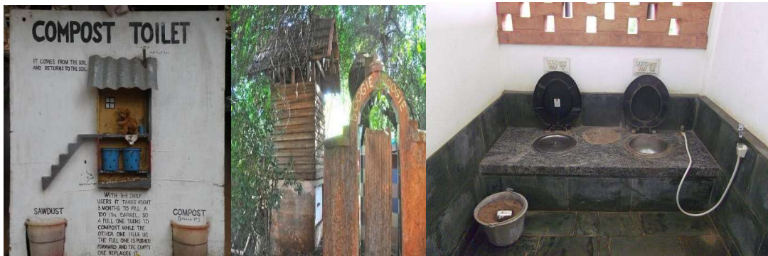
Figure 24. Compost Toilets in Fertile Forest and International House, Source: Personal and International House (International House 2011)
