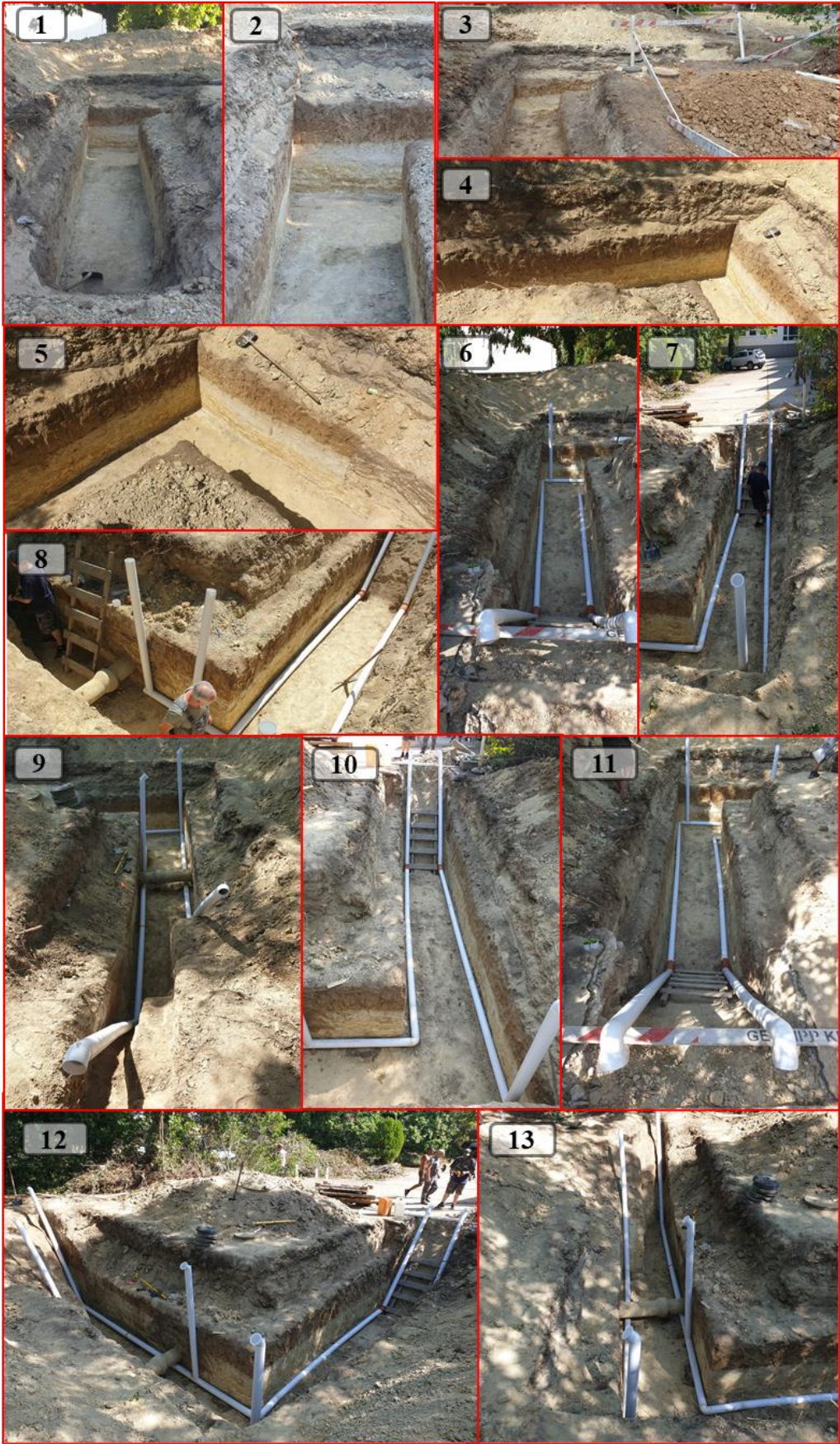
Fig. 9.1. Practical steps for digging the trench and laying the PVC pipes for installing the EAHE.
