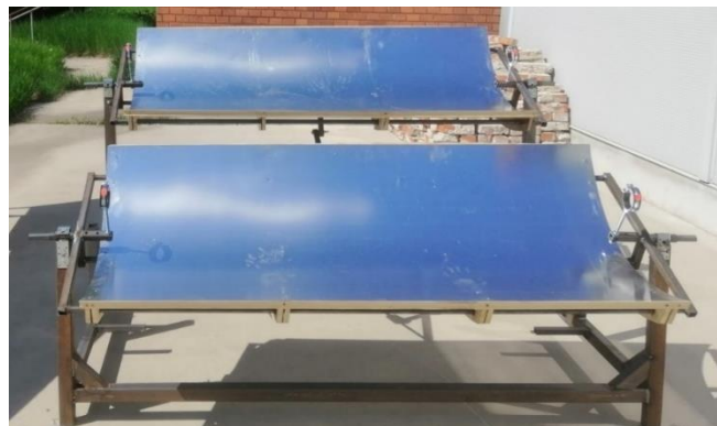
Fig. 3.5. Aluminium sheets reflective surface
