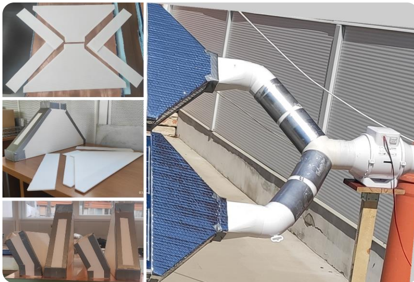
Fig. 3.20. Airflow ducts and pipes of the systems
